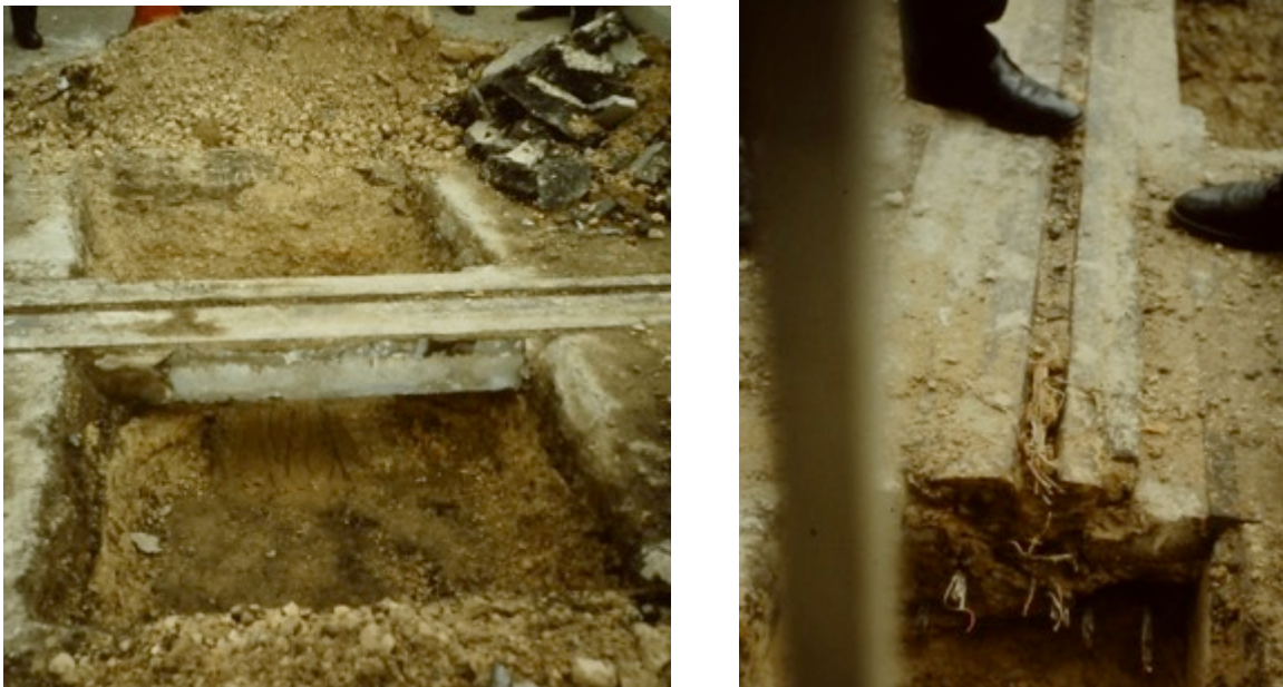
Fig. 15 After 1 million buses - LR55 excavated to examine condition
