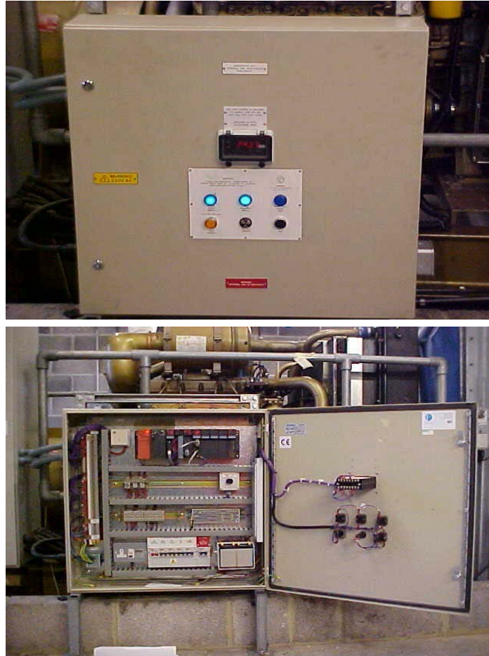
Load Management control panel, with the door open. Showing the PLC controller etc.
