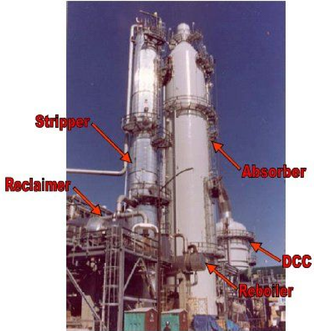
Bellingham Econamine FG SM Plant Ground View
