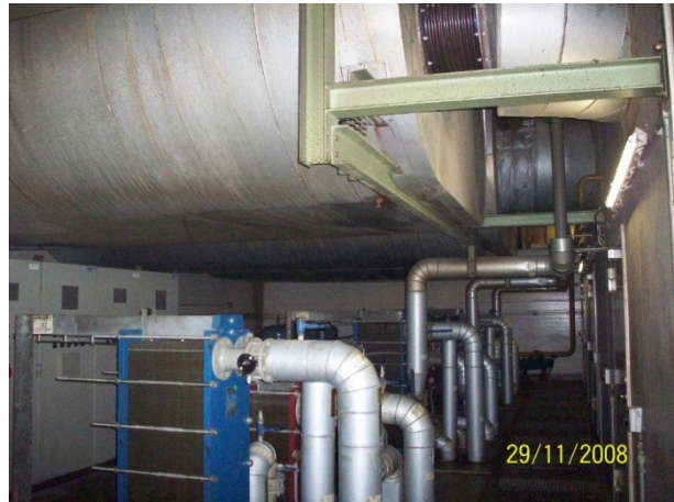
Engine water and oil cooling circuits showing plate heat exchangers and exhaust silencers above. The engine cells are to the left off the picture
