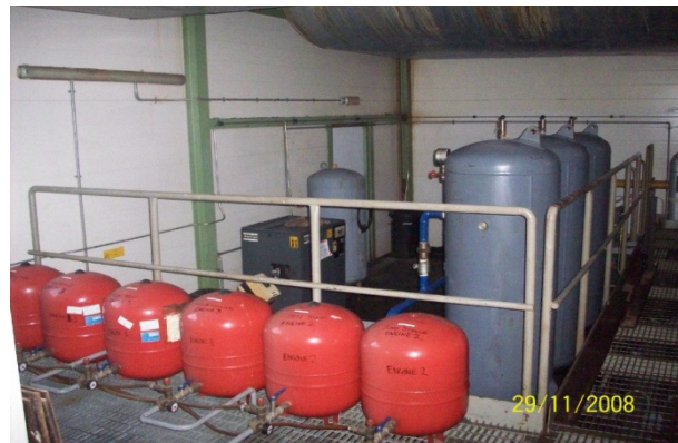
Air start equipment
