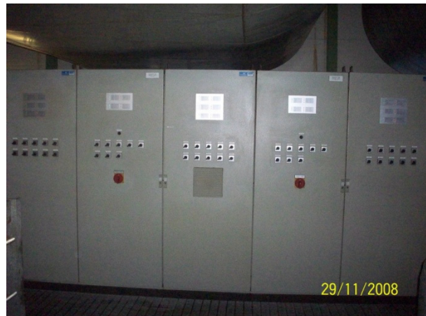
Five panel ABB 11000 volt switchboard with three genset incomers, one station transformer feeder and one mains outgoing breaker
