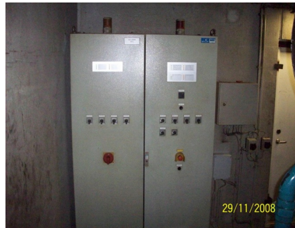
Generator control panels
